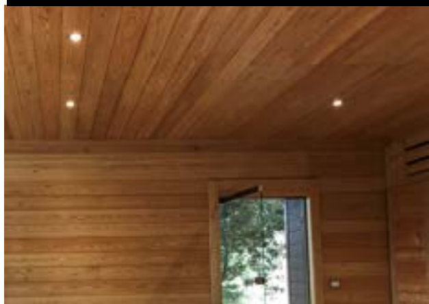
SPOT LED A SOFFITTO
